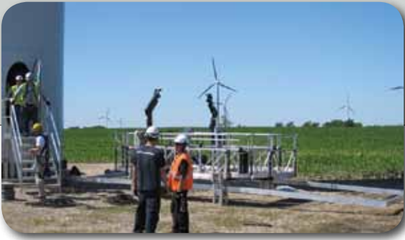
A maintenance crew has assembled a 360° platform and awaits a rigger in the nacelle to drop hoist lines. The black hoist arms on the platform guide the lift ropes away from the structure.
